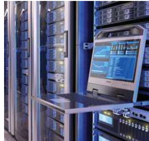
Server Room / Server Rack
