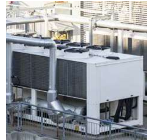
Chilled Water System
